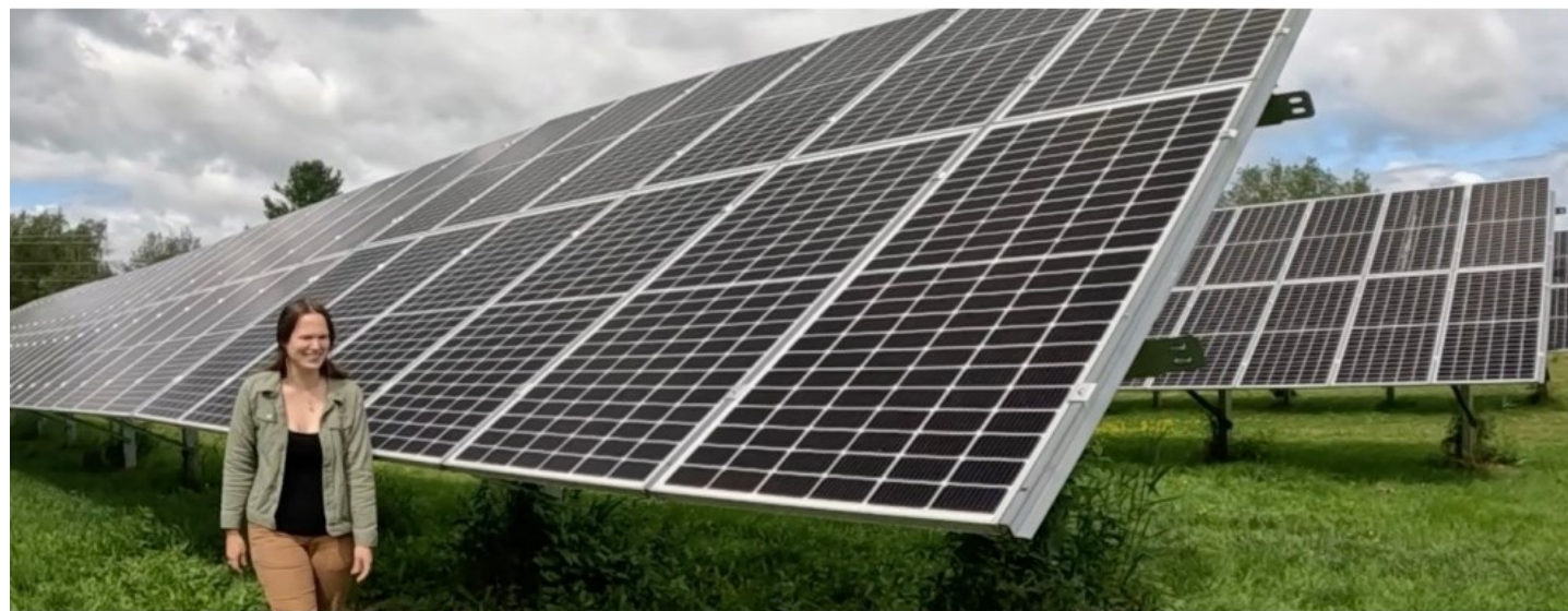
Energy Coordinator & Climate Change Specialist Jillian Wilde at Wastewater Treatment Plant microgrid
