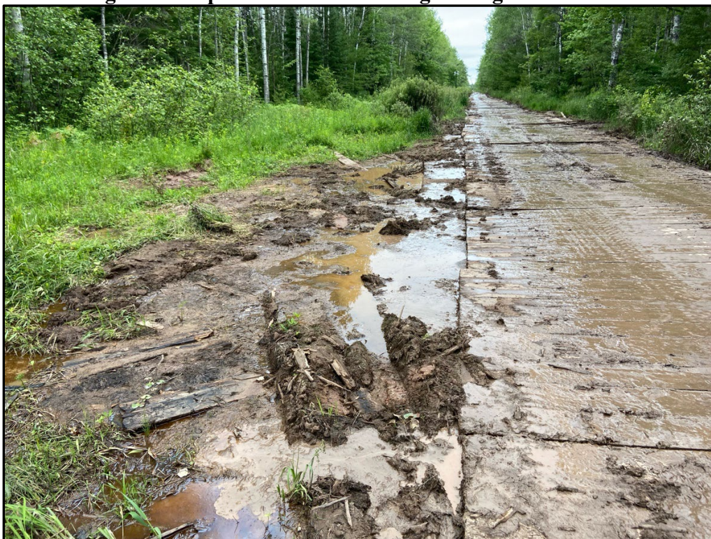
Fig. 3: Example of Wetlands Damage Along Access Route
