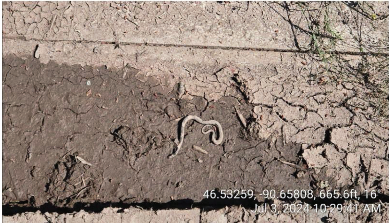
Figure 4. A dead snake alongside the construction matting used in Enbridge's Line 5 workspace. Snakes were observed by tribal staff as sunning themselves on construction matting—whether this snake was hiding or more obvious on top, it did not survive its encounter with the construction matting.
