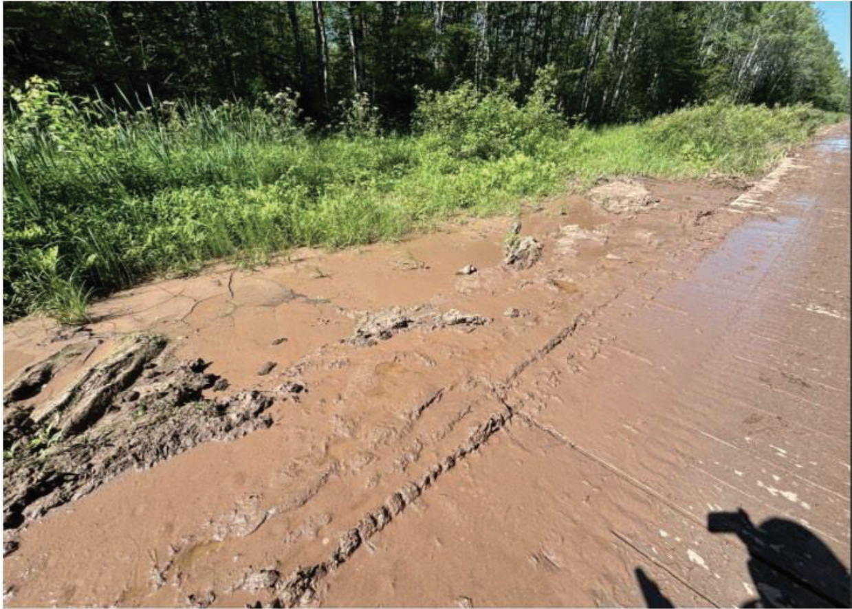
Figure 6. Soils being pushed out from under the construction matting and into adjacent wetlands as mats sink further into the soft substrate of the wetland, they were placed on top of from the vehicle traffic.
