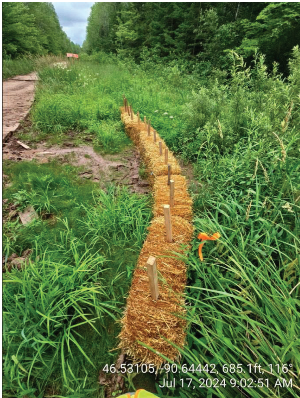
Figure 10. The photo shows the installation of straw bales to attempt to contain sediment from soils disturbed by the construction matting moving outside of the construction corridor and farther into the wetlands. Sediment deposits can be seen on both sides of the straw bales, indicating that either these sediment control practices were not implemented when they should have been, or they were not installed correctly.
