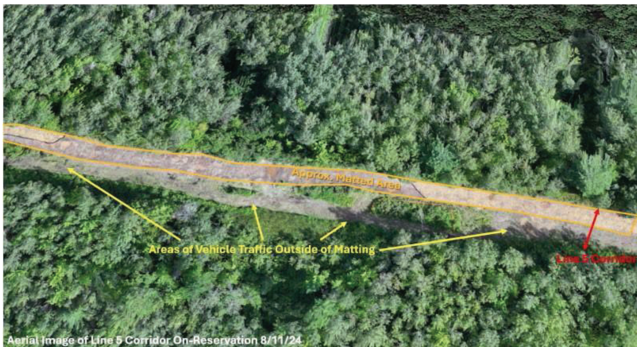
Figure 1. An annotated aerial image taken by drone over the Enbridge Line 5 corridor on August 11, 2024, shows a portion of the access route into a construction site where matting has been removed and some straw bales and sediment logs installed. Noted within the image are where the construction mats were placed per permit approval, the general width of Enbridge's Line 5 corridor, and areas where vehicle traffic clearly occurred not on the construction mats.
